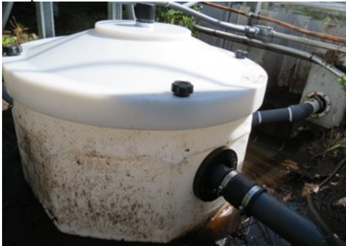
Photo (left) of a sump basin prior to construction of access docks around the sump. Photo (right) of a sump system prior to installation.
